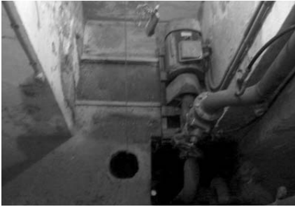
Figure 22. Pumping station supplying Ocaña with water from the qanat
